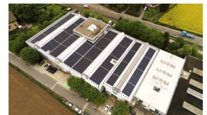
Photovoltaic panels produced 325,556 kWh in 2023, representing 10% of the consumption of the Kudelski Group Swiss HQ located in Cheseaux-sur-Lausanne.
