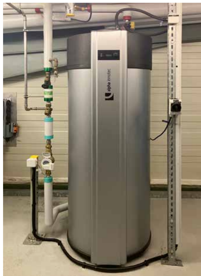
Swiss HQ, Cheseaux-sur-Lausanne: heat pump boiler installed to replace a classic electrical boiler.
